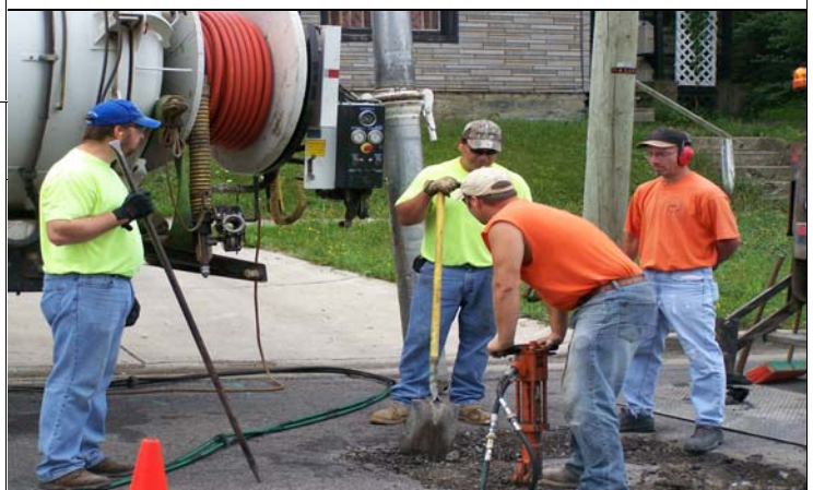
BPU Waste Water employees Bob Howe, Chris Calkins, Bob Sischo and Carl Spitale replace a manhole on Eighth Street. BPU Waste Water workers are involved in this aspect of high-way work performed in the City. Winter weather soon will bring such projects to a close.
