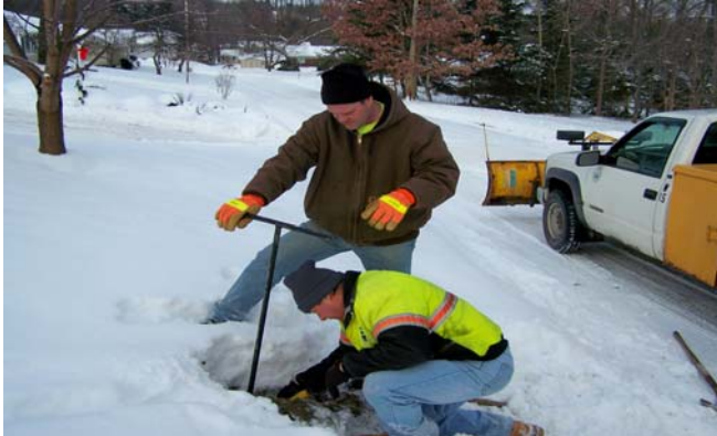
BPU water engineer Mike Saar and water service worker John Penna work to repair a water main break in the city.
