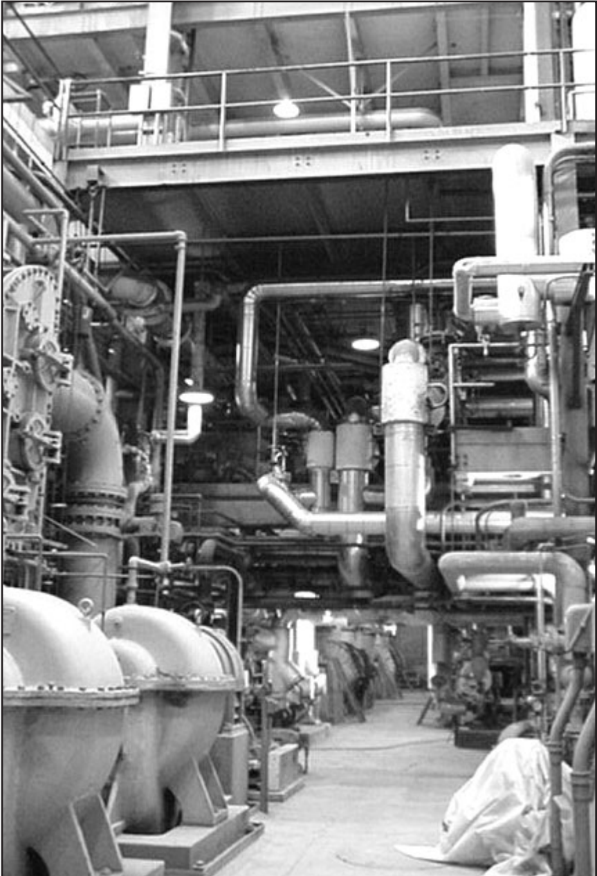
The floor of the Samuel A. Carlson Generating Station with the condensers in the left foreground looking toward the coal mills.
